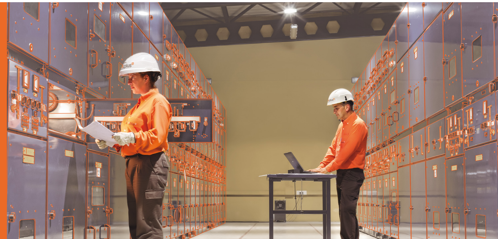
Electrical technical assistance developed at a substation
